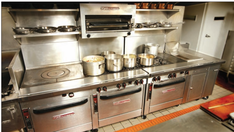
Paul Kahan, chef-owner of Blackbird in Chicago says the kitchen is more efficient since the installation of new cooking appliances, including a sectional range and a radiant heat salamander.
